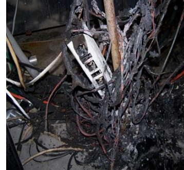
Fire is a potential hazard when using electrical equipment or wiring incorrectly.
