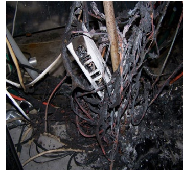
Fire is a potential hazard when using electrical equipment or wiring incorrectly.
